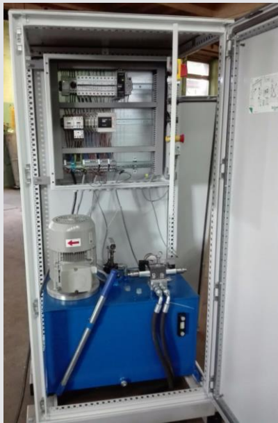
HPU + internal cabinet
